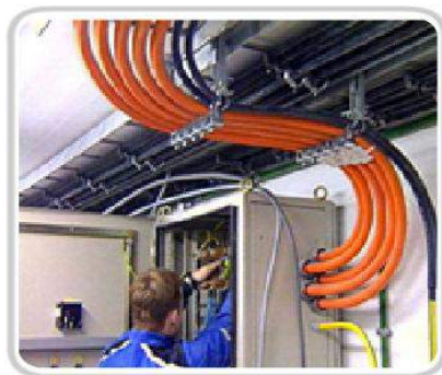
The separation of data and electrical power cabling must comply with safety codes.
