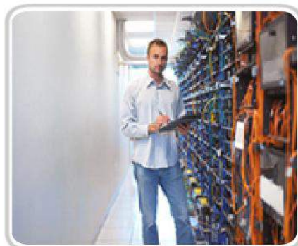
Installations must be inspected for damage.
